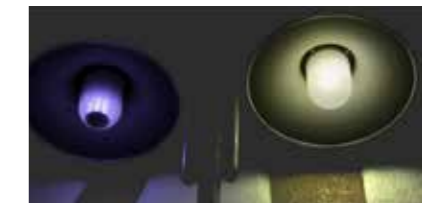
The darkening and blue drift of the lamp on the left indicates "burning" of the conversion phosphor of the LEDs due to overheating.
